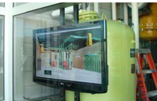
The deliberately exposed mechanical room and flat-screen TV displaying building data turns the entire building into a teaching tool, enabling students, faculty and visitors to not only learn about the inner workings of the school systems and energy usage, but to see their tax dollars at work.
